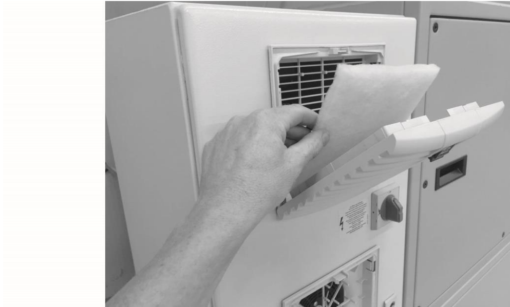
Fig. 130: Filter replacement in control cabinet
