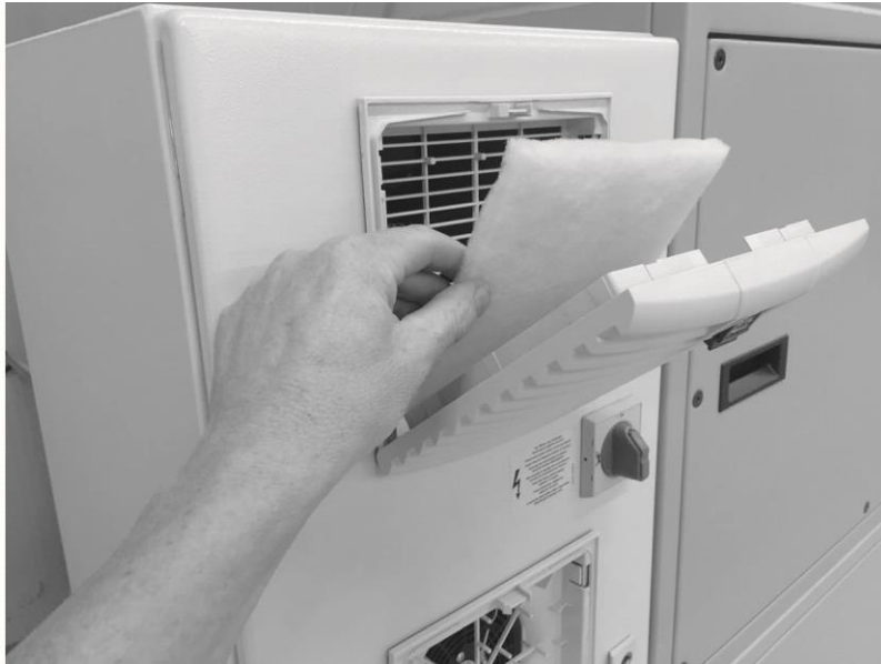
Fig. 99: Filter replacement in control cabinet
